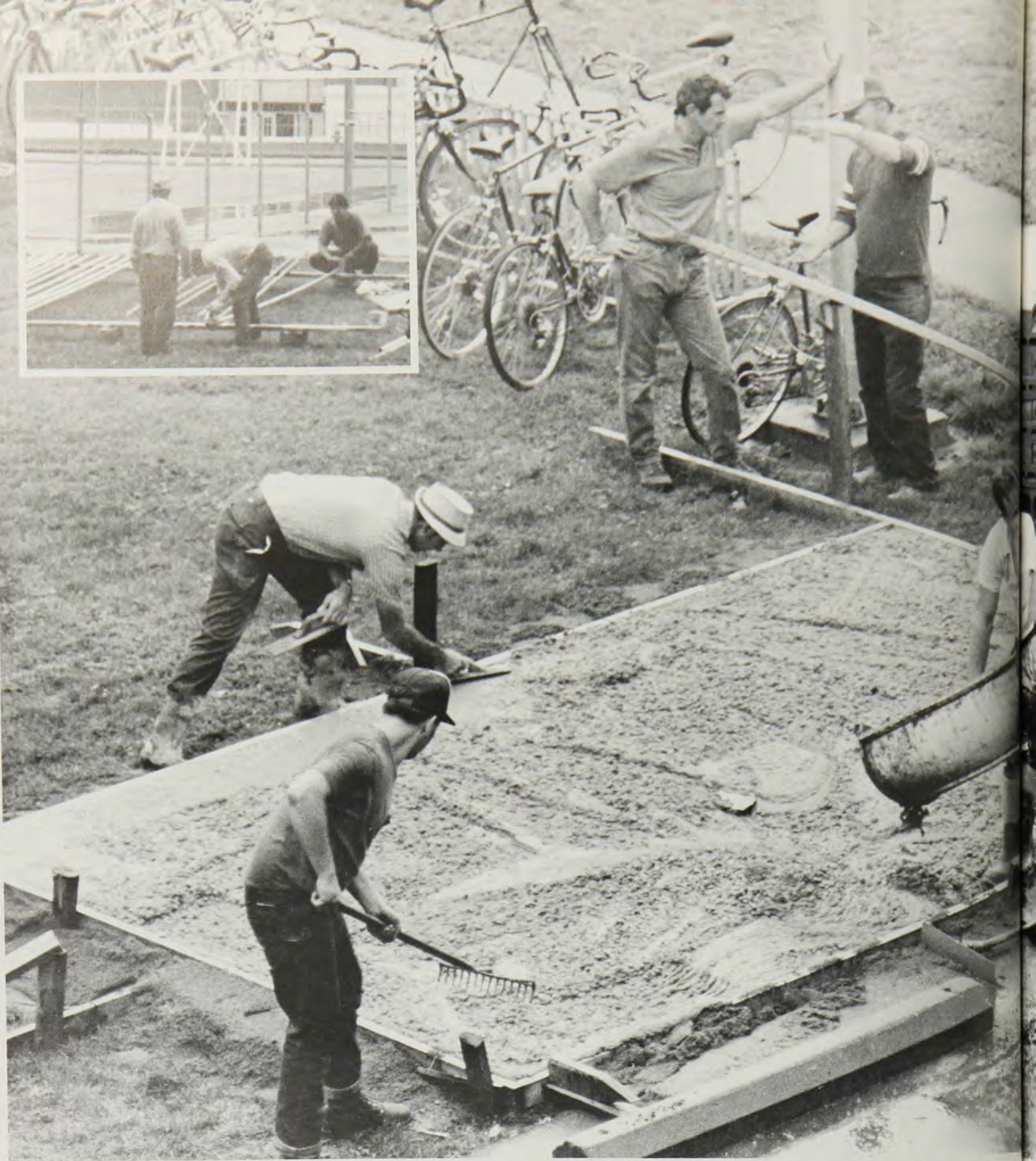
(Above, inset) Amid the drizzle and puddles, Bona workers construct the fence posts for the new tennis courts behind Rob-Fal.
